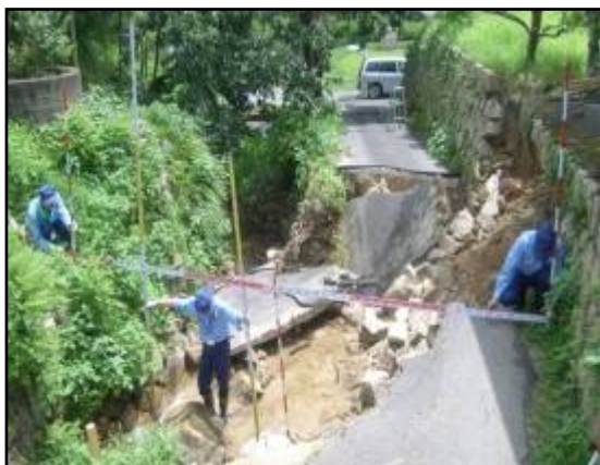
Figure 10. Damage assessment on the ground
